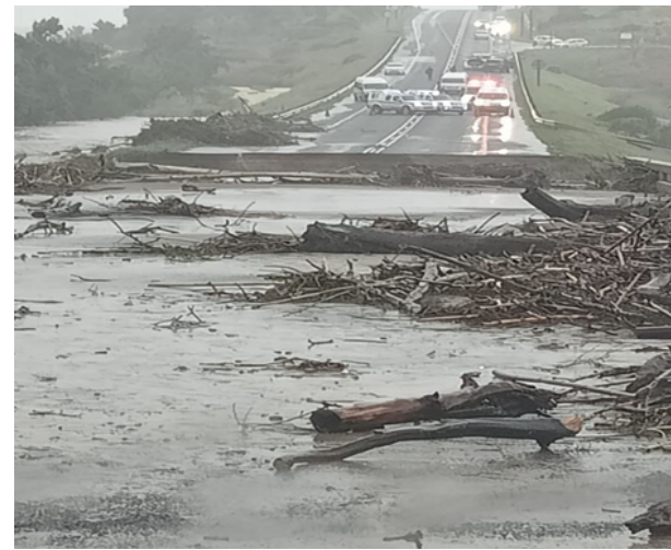
Infrastructure Destroyed Due to Heavy Downpours In Western Cape, South Africa □ 24th September, 2023
